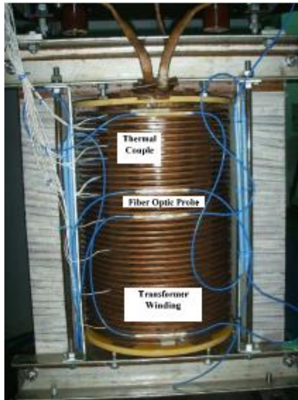
Figure 10: Exprimental setup of transformer with sensor and fiber optic core
